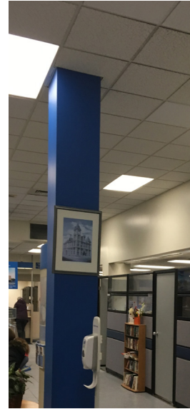
Interior column within central area of bank building, clad with drywall or plaster and painted.
